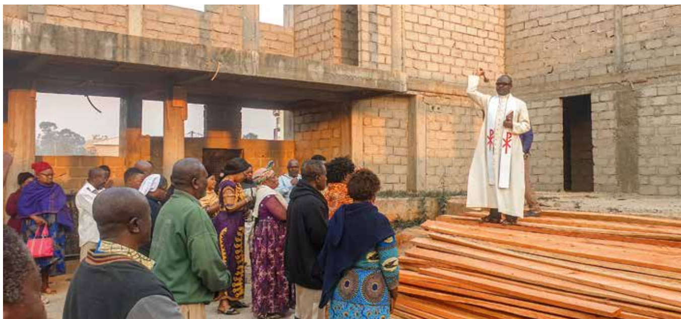
Blessing to mark the beginning of the roofing of the multi-purpose hall of St John the Baptist in Nkwen, Bamenda.
